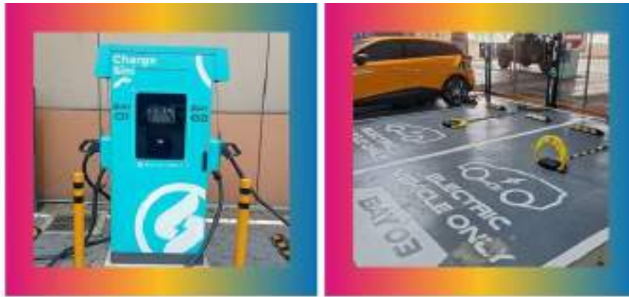
EV chargers available on our parking premises
